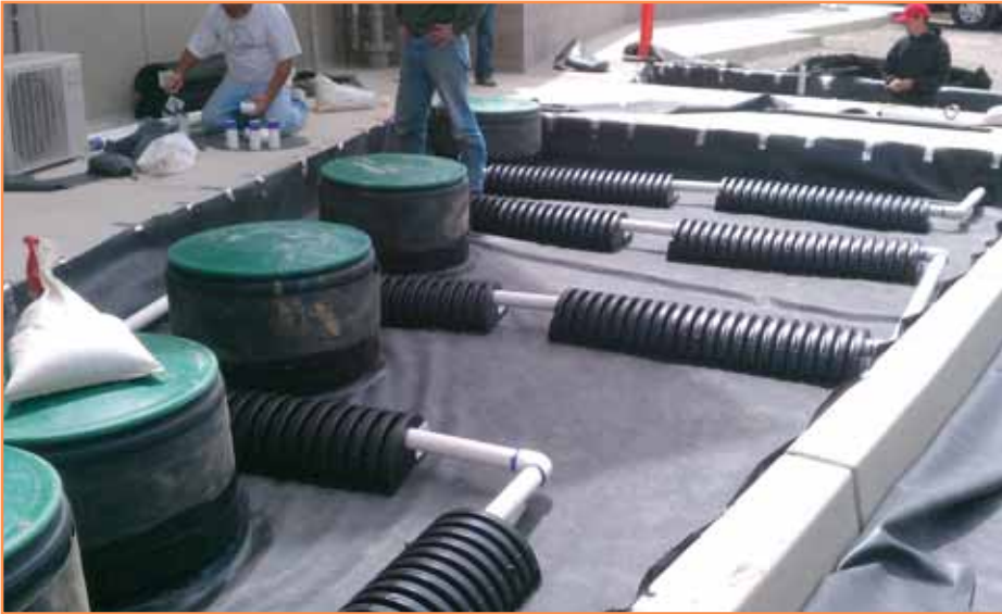
Installation of septic system and leach field chambers. (Photo credit: Chad Kennedy)
