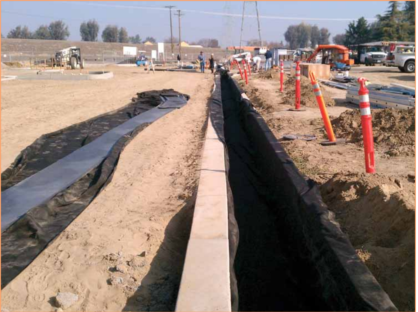
Installation of trench and chambers to collect all stormwater surface flow from parking lots and walkways. (Photo credit: Chad Kennedy)
