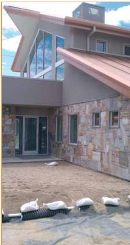
Veterinary hospital entrance during construction. Each layer of the system profile is visible. (Photo credit: Chad Kennedy)
